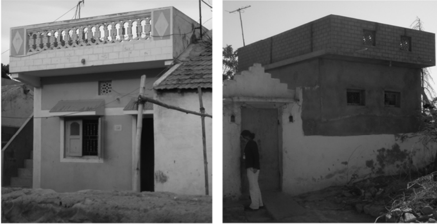
Figure 18.4 Examples of flat roofs with cantilevers (left: the slum community of Kajlinagar, right: the community of Bhimraonagar. Photos: J. Wendel).
